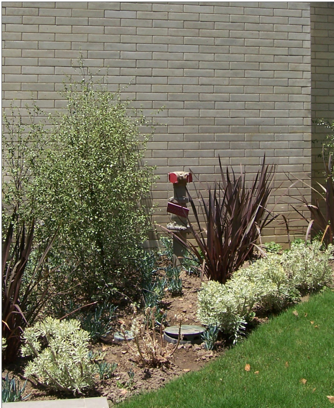
A back flow preventer that abuts the building and is screened from the view of the sidewalk and street by shrubs.
